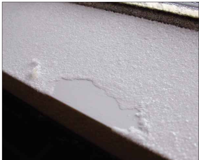
Heavy frost accumulation on this curtain wall sill illustrates the negative impact of perimeter thermal bridging on condensation resistance.
